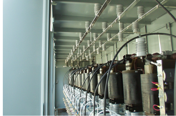
Figure 1: Typical Iron-Core Reactor Installation
