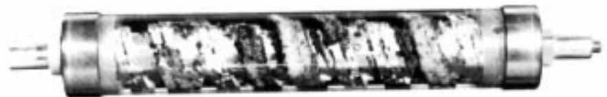
Figure 13. Fulgurite formation caused by a low fault current.
